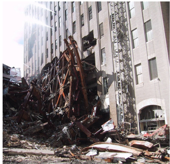
The damage to 140 West St was extensive
