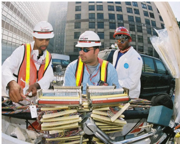
Every 3600 pair cable had to be respliced.
