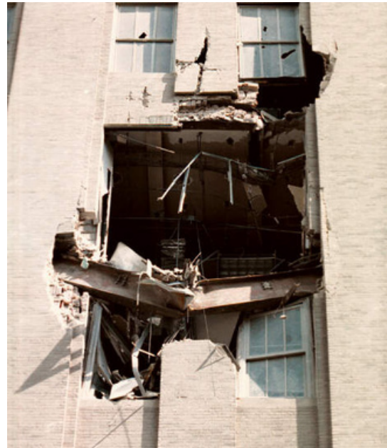
140 West Street, hit by debris from 7 WTC
