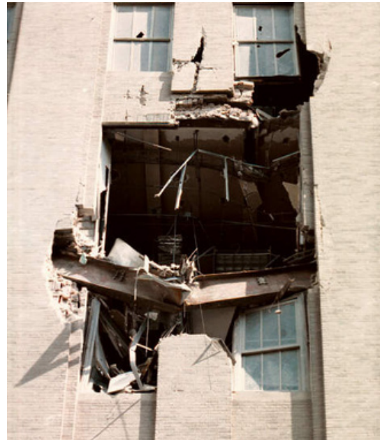
140 West Street, hit by debris from 7 WTC
